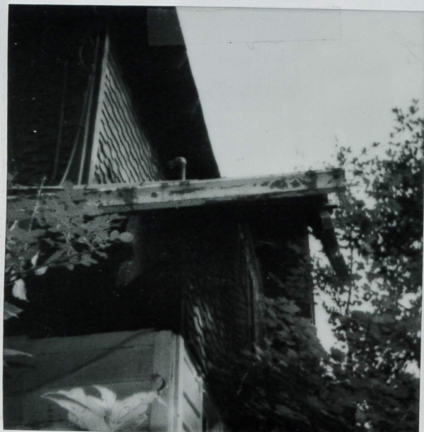
Rear 1402 showing ends "skewed" & bad cond.
