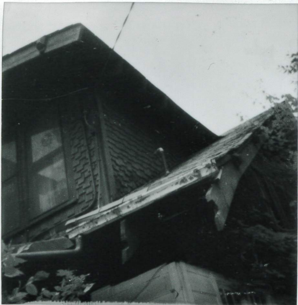
Other side rear 1402 Showing broken, crooked & sawed rafters
