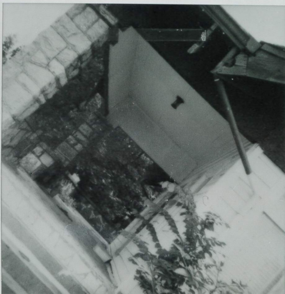
Another side view 1402 showing poor roof structure + badly sunken porch (Before)
