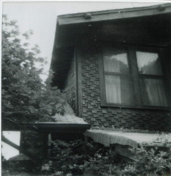
Rear 1402 Showing poor const. rear porch & sawed rafters plus crooked construction
