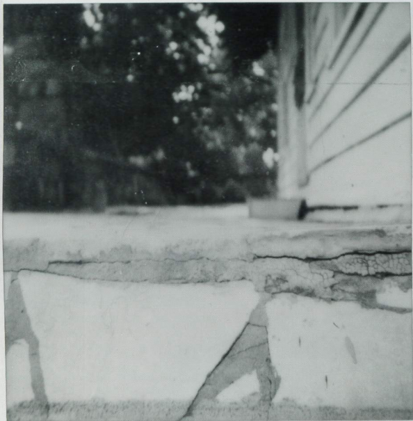
Side 1402 showing 6" drop in porch - wrong direction (Before)
