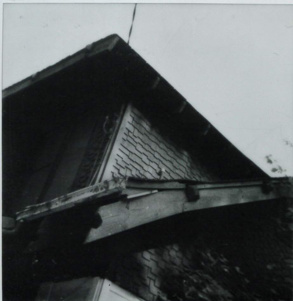
Rear, 1402 showing rotten, sawed and broken rafters (Before)
